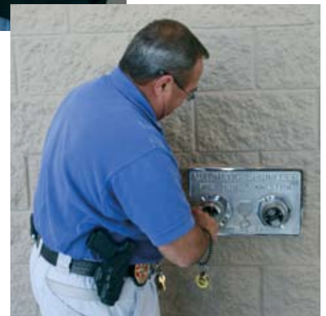
Deputy Fire Marshal Terry Aikman installing locking FDC plugs on a new Lowes Home Improvement store's standpipes.
